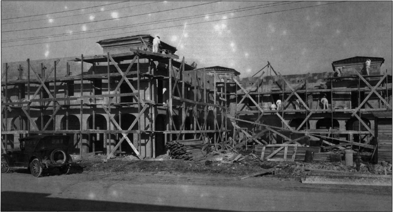
The Bay Isle Building under construction on East Davis Boulevard on Davis Islands, January 13, 1926. (Photograph courtesy of the Tampa-Hillsborough County Library System, Burgert Bros. Collection)
